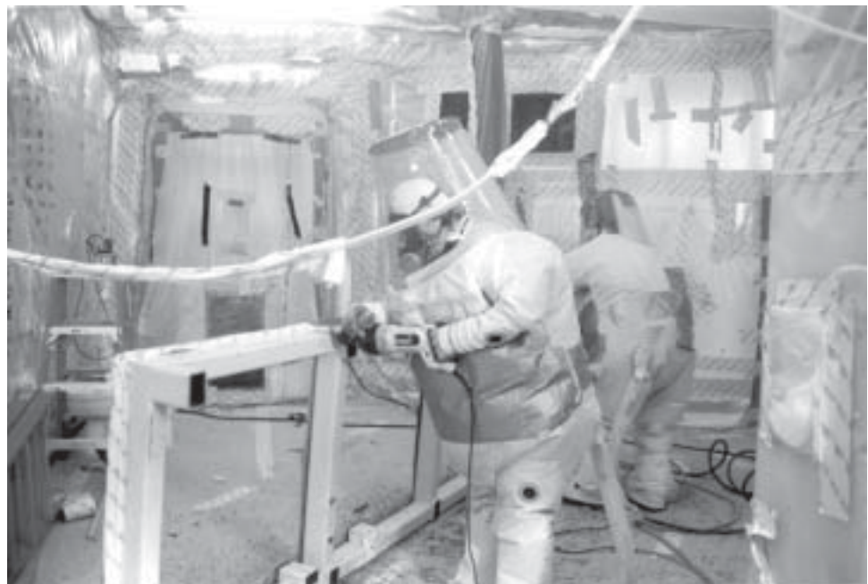
Plutonium contamination requires the wearing of safety equipment as buildings are demolished.
