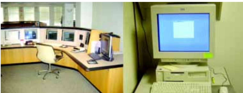
Figure 4.14. A SCADA console is shown on the left with a simulator on the right indicating that simulators need not be exactly the same as the SCADA console.
