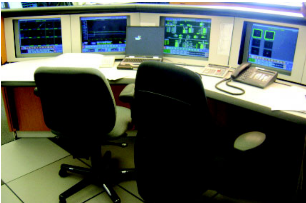
Figure 1.1. View of a SCADA workstation showing arrangement of screens and input keyboard.
