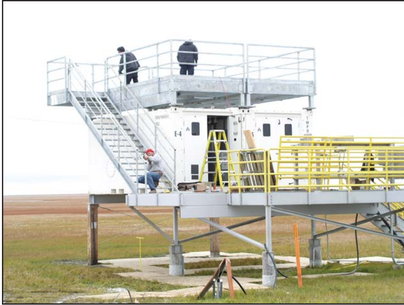
Additional instrument shelters and topside deck for “visiting” upward-looking instrumentation installed at the Barrow, North Slope of Alaska ARM Climate Research Facility during FY 2005.
