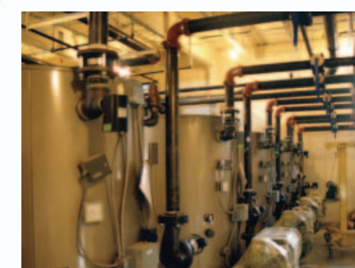
Five natural gas-fired boilers are more efficient than a traditional mega-boiler, since individual boilers can work more often in their highest efficiency ranges.
