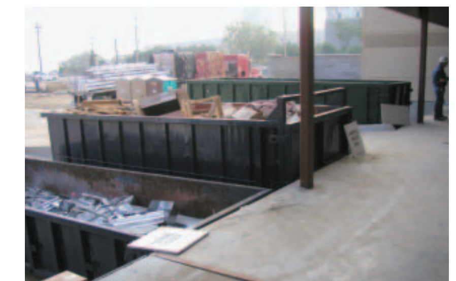
The lab design team implemented a construction waste recycling plan for concrete, metals, wood, asphalt, and paper. The team was able to divert 72 percent of construction debris from area landfills.
