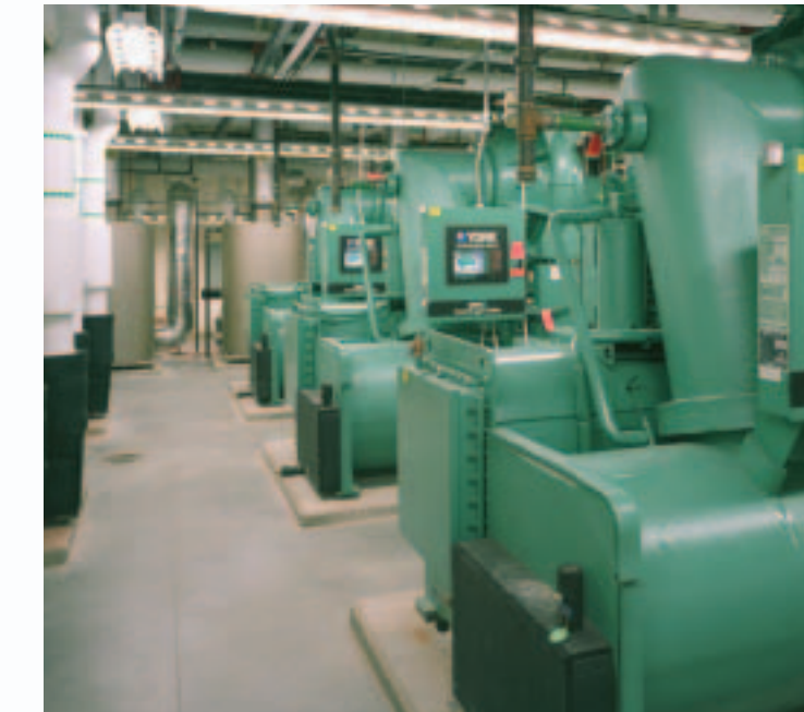
By coupling a variable frequency drive chiller with two conventional chillers, the lab is able to maximize efficient chiller operations over the range of cooling needs.
