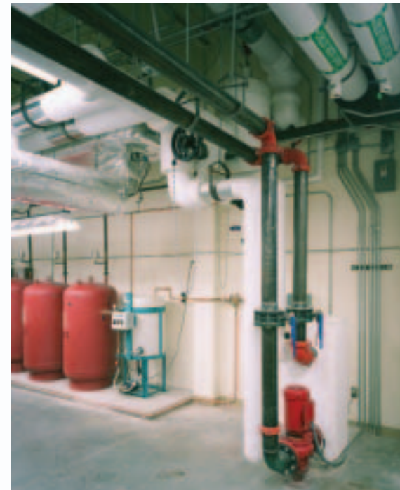
A plate and frame heat exchanger system was added to the initial design after energy modeling revealed additional energy efficiency opportunities.
