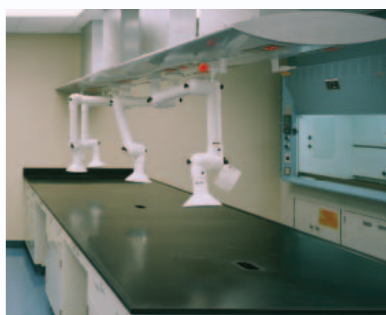
Sophisticated variable air volume (VAV) fume hoods and systems allow ventilation, cooling, and heating requirements to be reduced when hoods are closed, at night, and on weekends.
