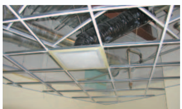
During construction, the HVAC system and duct work were sealed on a daily basis to prevent infiltration of any dust, chemicals, or odors due to construction. Before occupancy, the system was flushed and fresh air filters were added.
