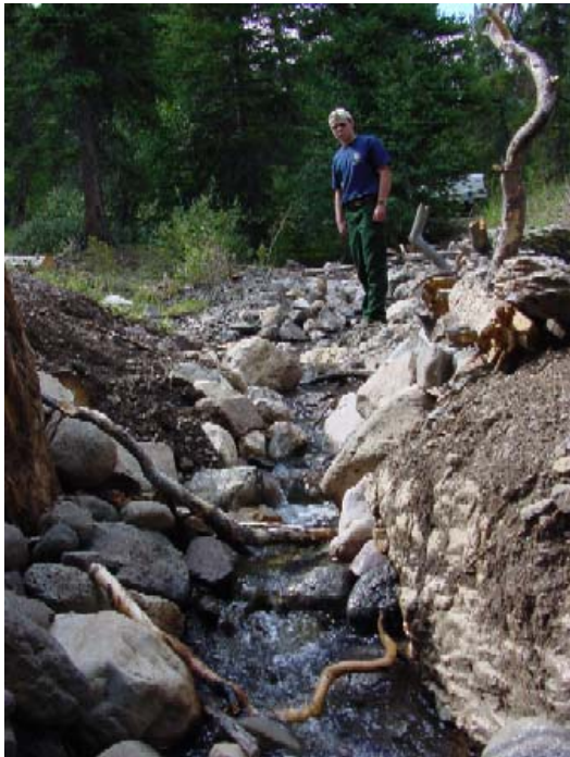
Figure 7. Newly constructed stream channel that bypassed the barrier and restored fish passage.
