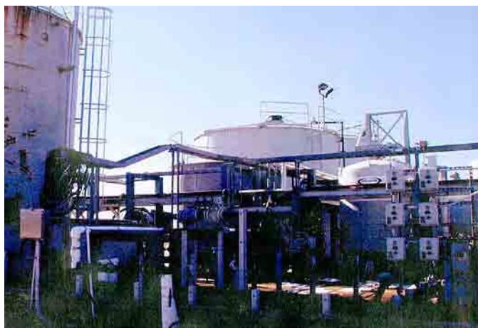
The aging groundwater treatment plant needs to be replaced.
