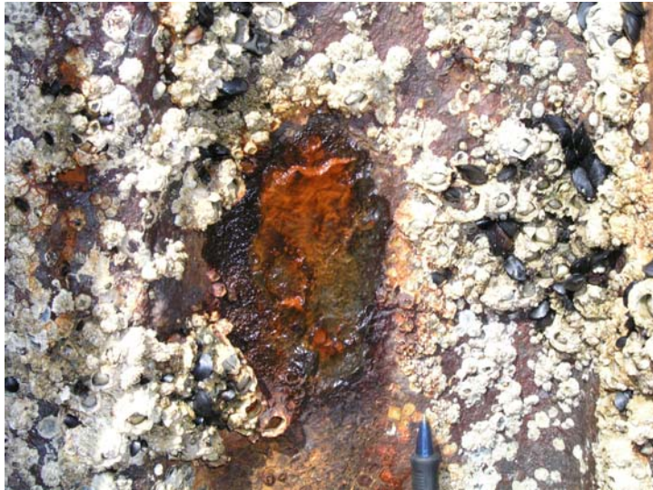
Photo 11. Corrosion and seep on outside of sheet pile wall.
