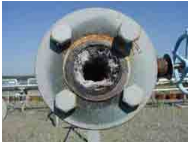
The chemical naphthalene clogged the pipes. Note the crystals in the inner ring.
