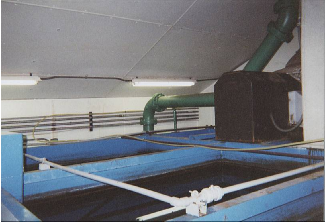
Figure 4-2. Top View of Pre-Existing Gravity Filter Cells (with Two of Four Cells Shown)
