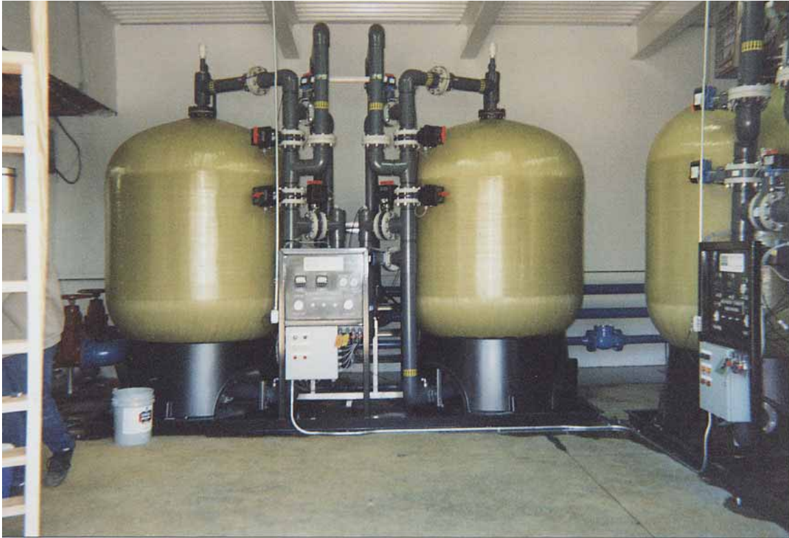
Figure 4-6. Photograph of the Two APU-300 Units at the Brown City Site
