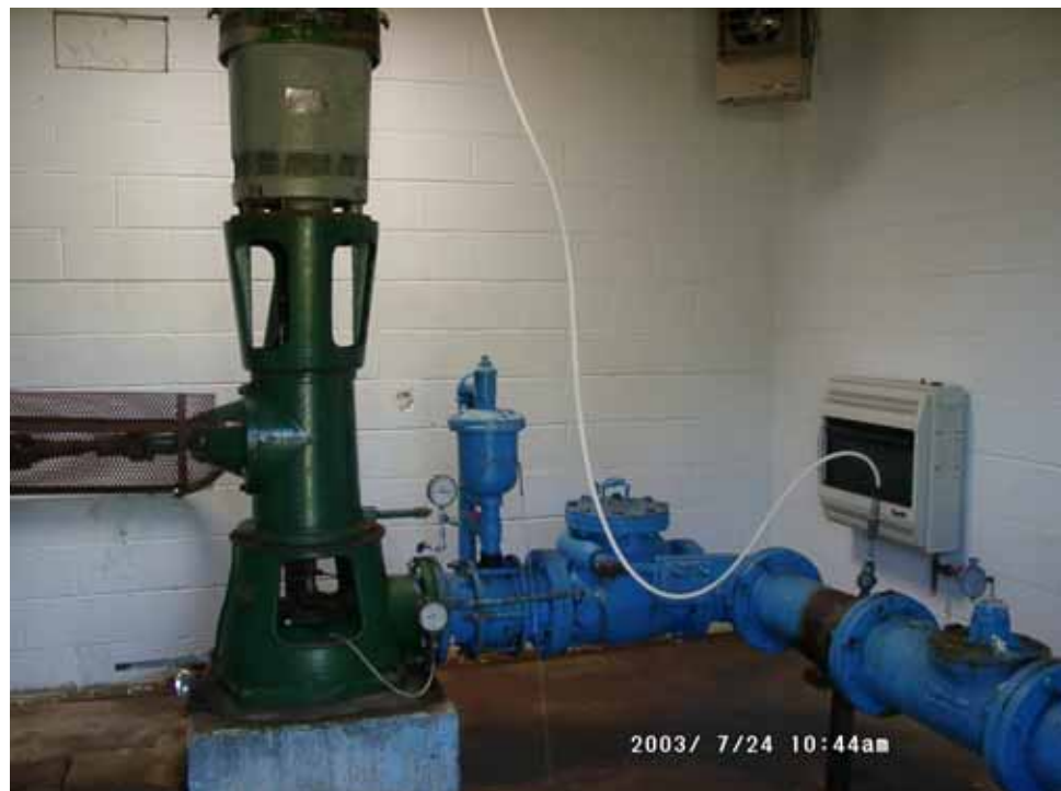
Figure 4-3. Pump Motor, System Piping, and Chlorine Addition Assembly at Wellhead No. 4
