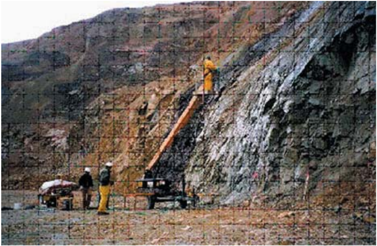
Figure 4-2. Spray application of the EcoBond technology onto the GSM highwall at Plot C.
