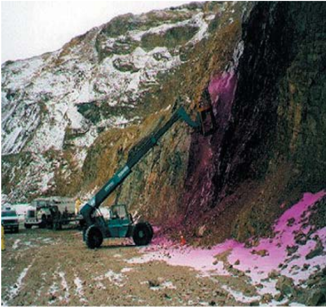
Figure 4-4. Spray application of the UNR/KP technology on the GSM at Plot E.
