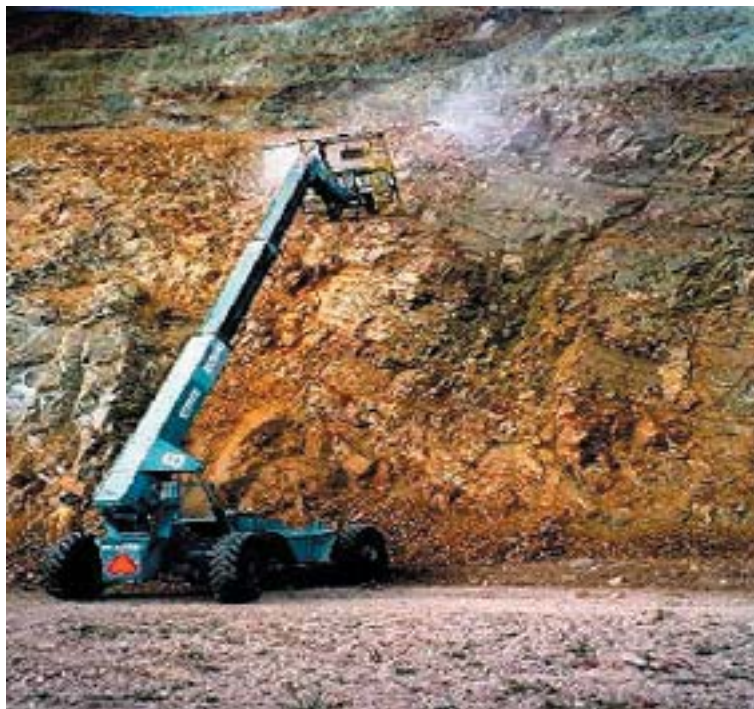
Figure 4-3. Field application of the UNR/MgO technology on the GSM highwall at Plot D.
