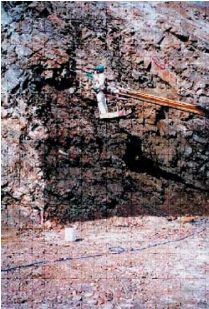
Figure 4-1. FARS being spray applied on the GSM open-pit highwall at Plot B.
