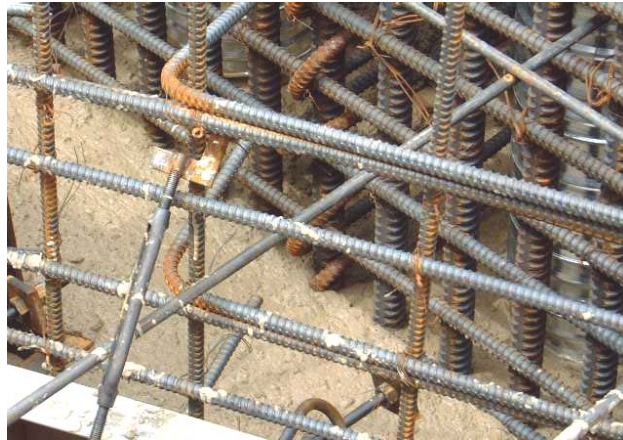
Photo 2 Condition of Concrete Flowing 4
