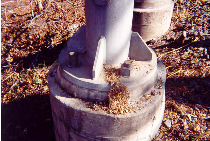
Figure A3 Missing Anchor Nut. If Span structure, rate as 2, Priority Repair 2. If Cantilever structure, rate as 3, Priority Repair 1.
