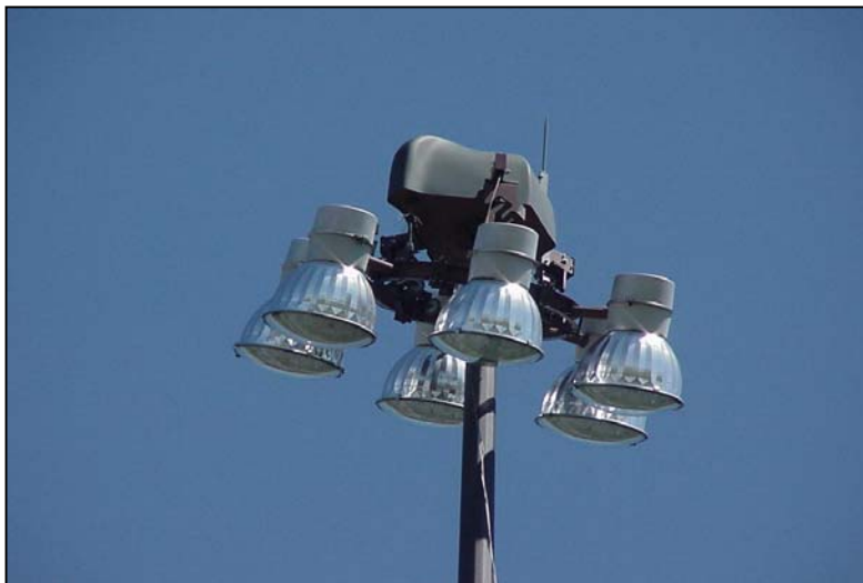
Figure 30. Misaligned Luminaire Ring.
