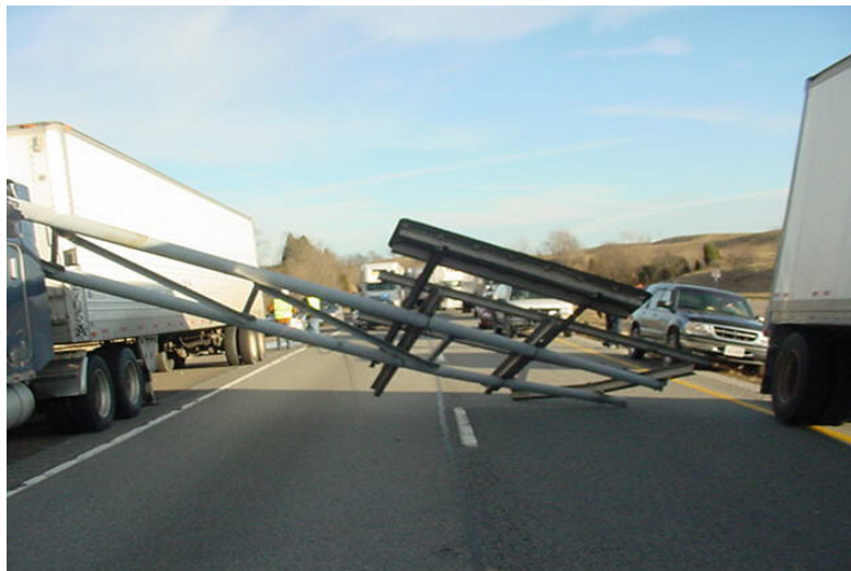
Figure 1. Cantilever Sign Structure Failure.
