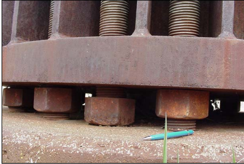
Figure 28. Loose Leveling Nuts on a High Mast Structure. (Note: Top Nuts on Chairs Out of Photo)
