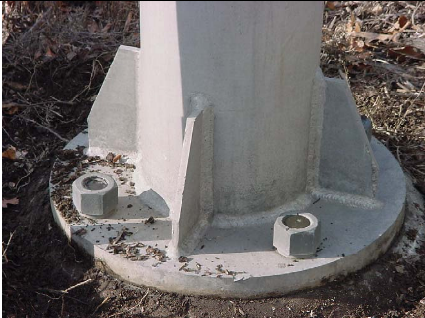
Figure A4 Anchor rods not fully engaged. If 80% threaded, note on report, rate S.02 as '1', no repair. Loose Nuts (Washers Slip) Less than 50% slip, rate S.02 as '2', Priority Repair 2. More than 50% slip, rate S.02 as '2', Priority Repair 1.
