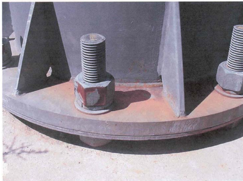
PHOTOGRAPH 5: LIGHT CORROSION ON BASE PLATE
