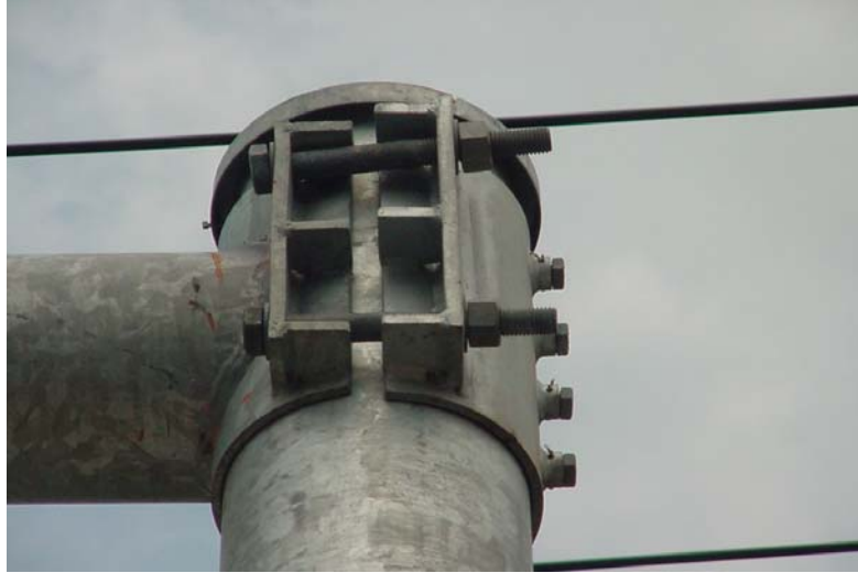
Figure 27. Post to Arm Connection Showing Poor Fit-Up Due to Use of Incorrect Components.
