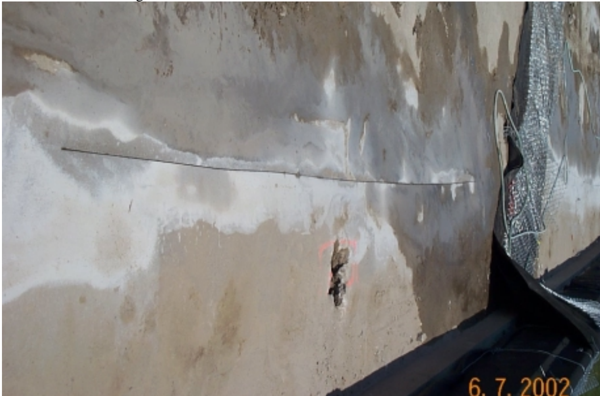
Attachment 12 – Longitudinal saw cuts in the deck
