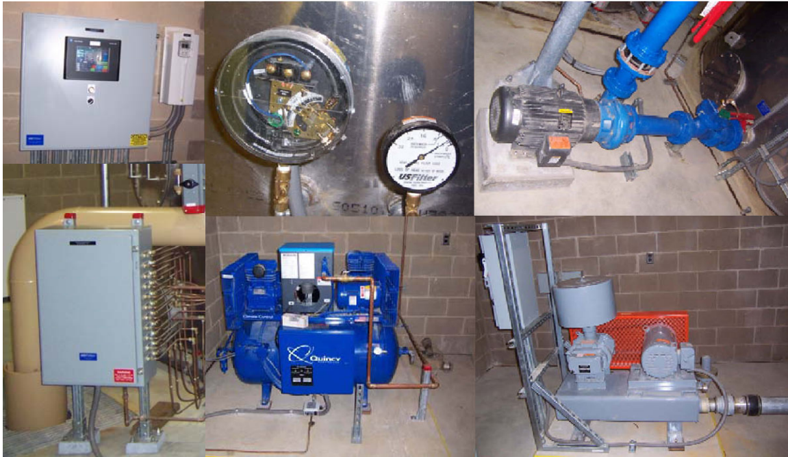
Figure 4-6. Control Panel and Ancillary Equipment
