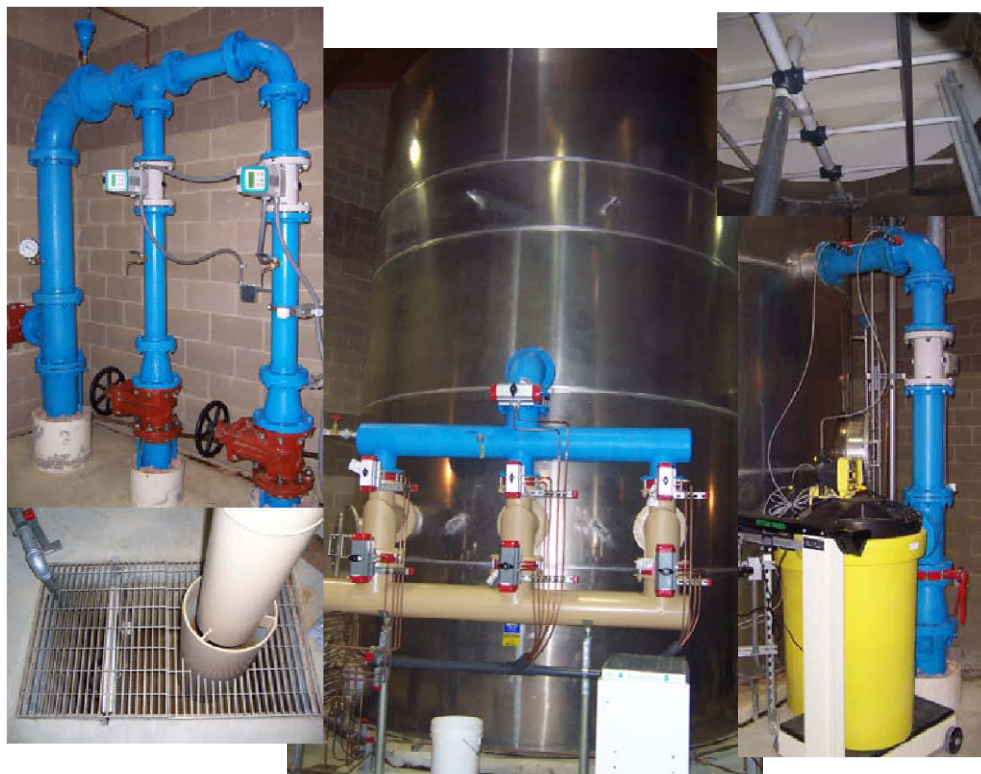
Figure 4-5. Treatment System Components
