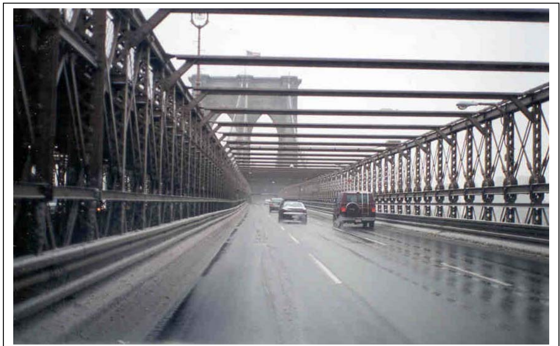
Photo Exhibit G: Pavement condition after DOS applied salt. (Note: Photo D illustrates the pavement condition before salting occurred (1/14/99).
