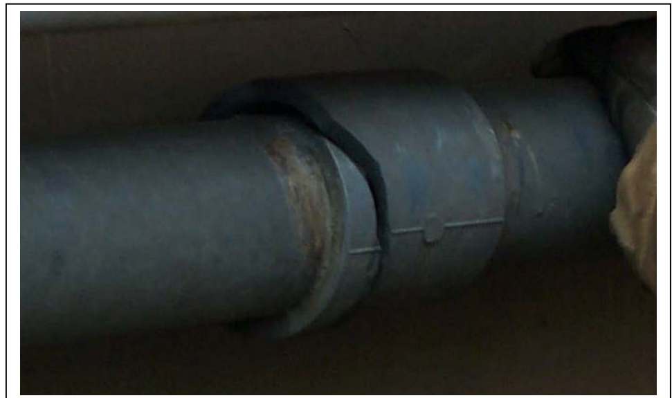
Photo Exhibit I: Typical joint failure
