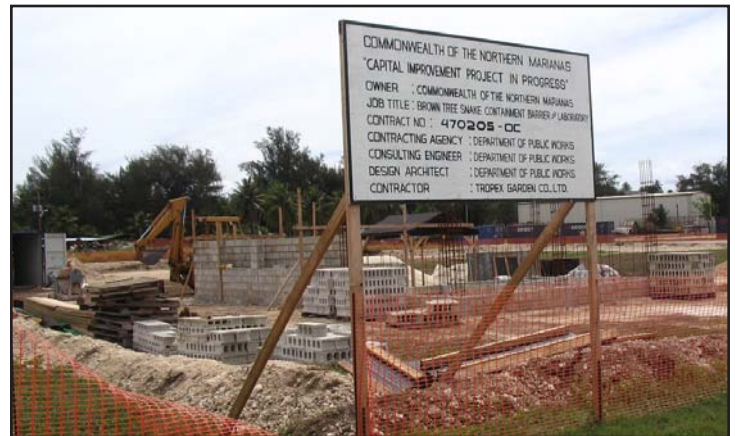
Containment barrier for brown treesnake ( Boiga irregularis ) during construction. Photo courtesy of Nate Hawley.
