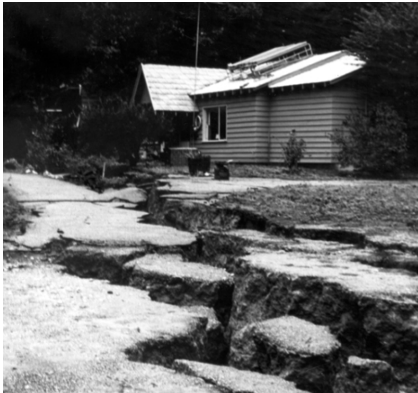
Loma Prieta, California, Earthquake October 17, 1989. Crack system near Summit Road, half a mile southwest of Highway 17. View is northwest. A wide zone of dominantly extensional cracks passes several feet in front of the house. Figure 10-A, U.S. Geological Survey Circular 1045. Circular-1045 ( http://130.11.57.28/ci1045.htm ), Digital File:pla00036, ID. Plafker, G. 36
