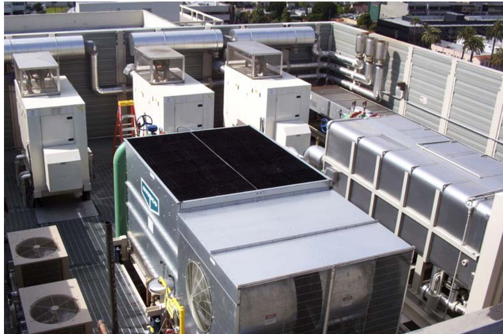
600 kW Plant with Absorption Chiller
