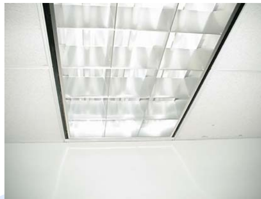
Lighting and Occupancy Sensors
