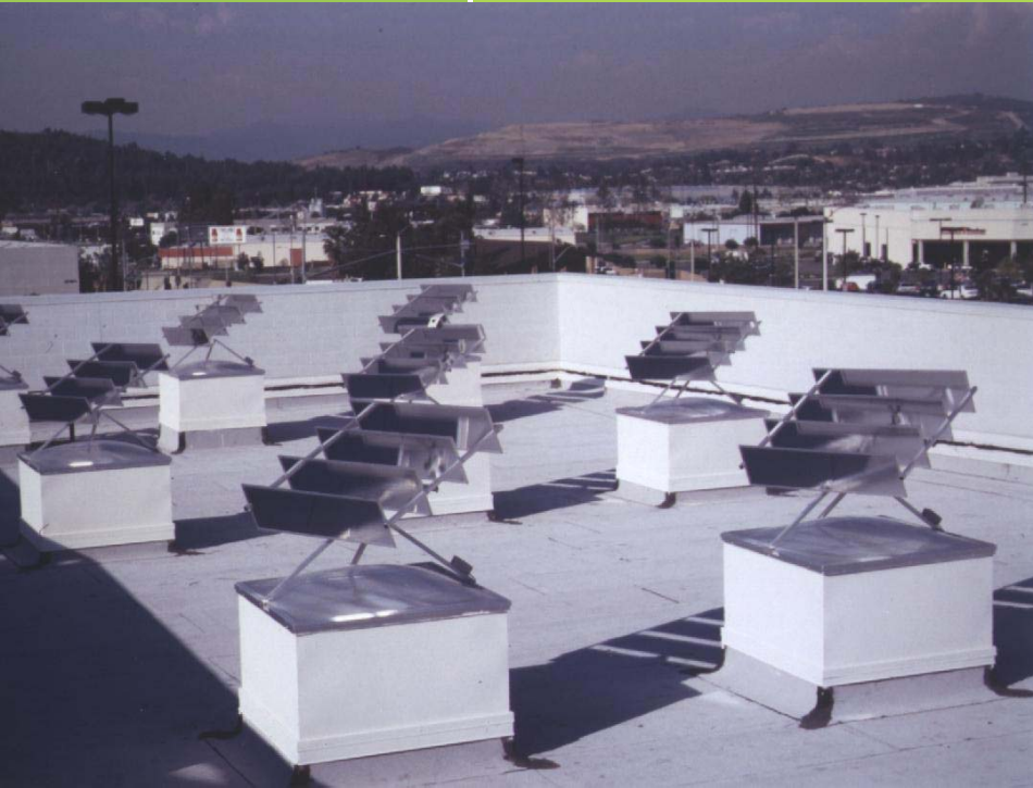
First version of a solar tracking skylight test and evaluation in City of Industry, CA-1993
