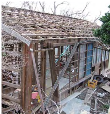
Roof Destroyed by Volcanic Gas
