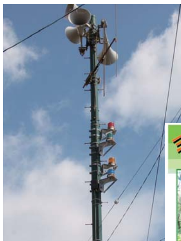
The Community Wireless System's Outdoor Loudspeakers with Revolving Lights
