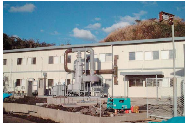
Desulphurization Equipment Installed in Accommodations
