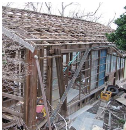
Roof Destroyed by Volcanic Gas
