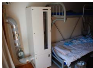
Fig. 9. Desulfurization equipment in a hotel.
