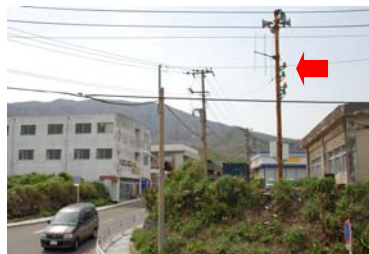
Fig. 7. Warning lights and speakers.
