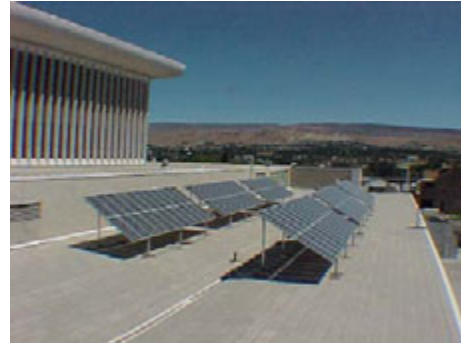
Photovoltaic panels at Wenatchee, Washington
