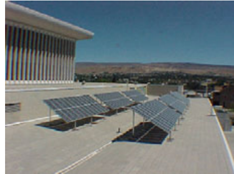
Photovoltaic panels at Wenatchee, Washington
