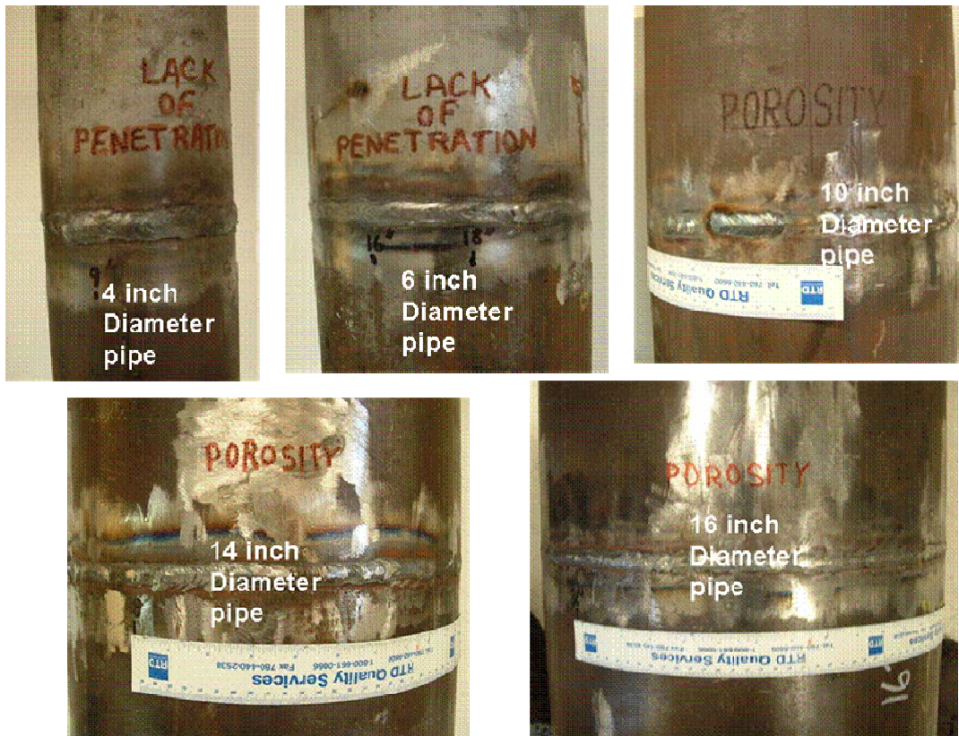
Figure 5. Photographs of portions of each pipe size showing some types of defects generated in the welds
