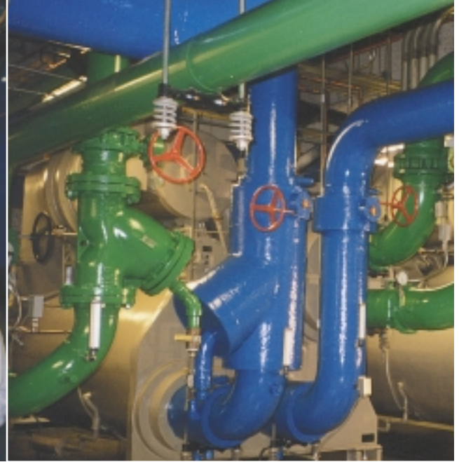
A shot taken in the central plant serving the building.
