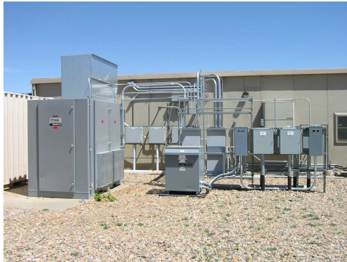
Figure 7. 165-kW Titan load bank (on left)
