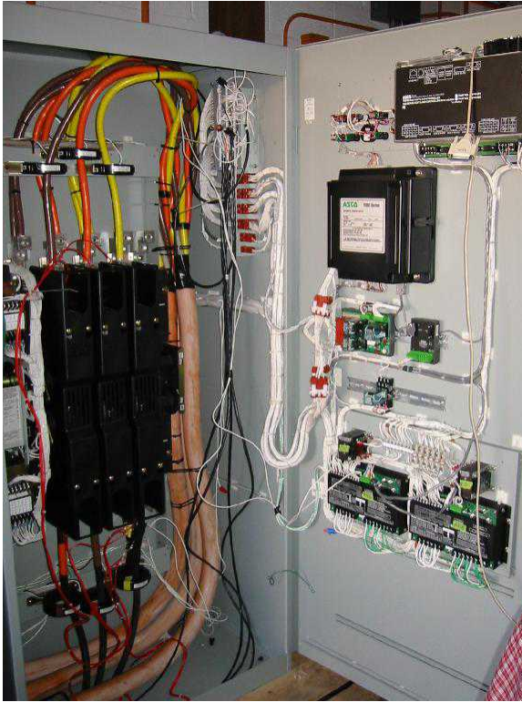
Figure 4. ASCO SLTS interior
