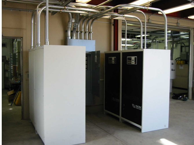
Figure 6. 200-kW grid simulator array
