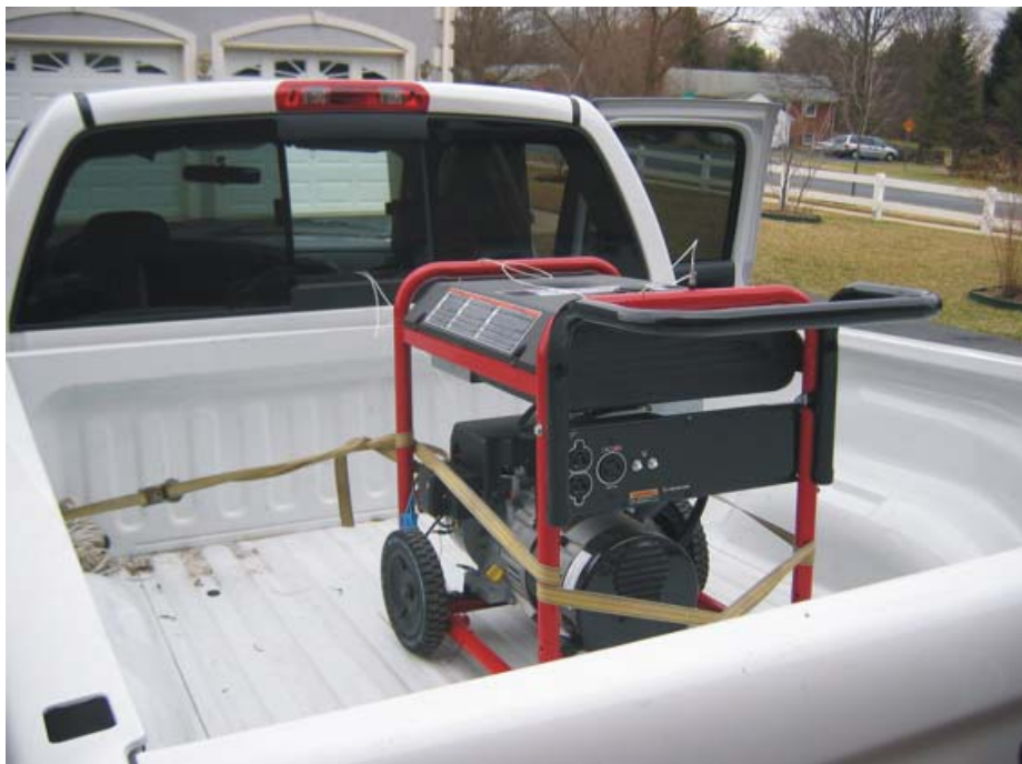
Figure 35. 5250 Watt Generator in the Pick-up Truck
