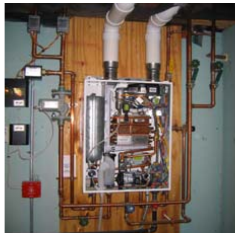
Figure 19. Installed combination boiler
