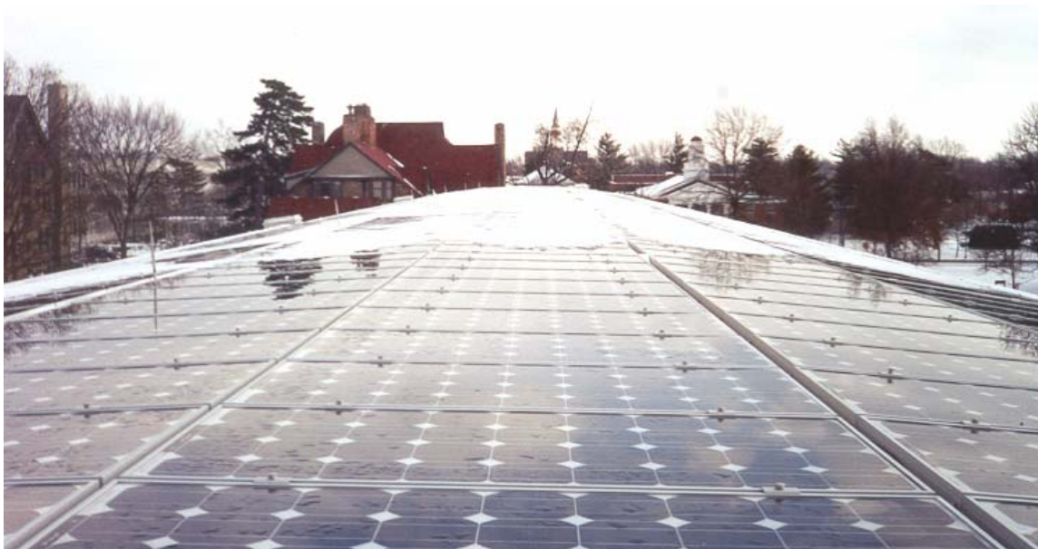
Figure 3-38 Oberlin PV array partially covered with snow
