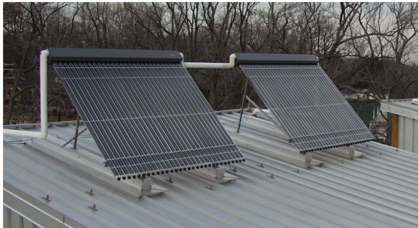
Figure 3-49 CBF evacuated-tube solar collector arrays
