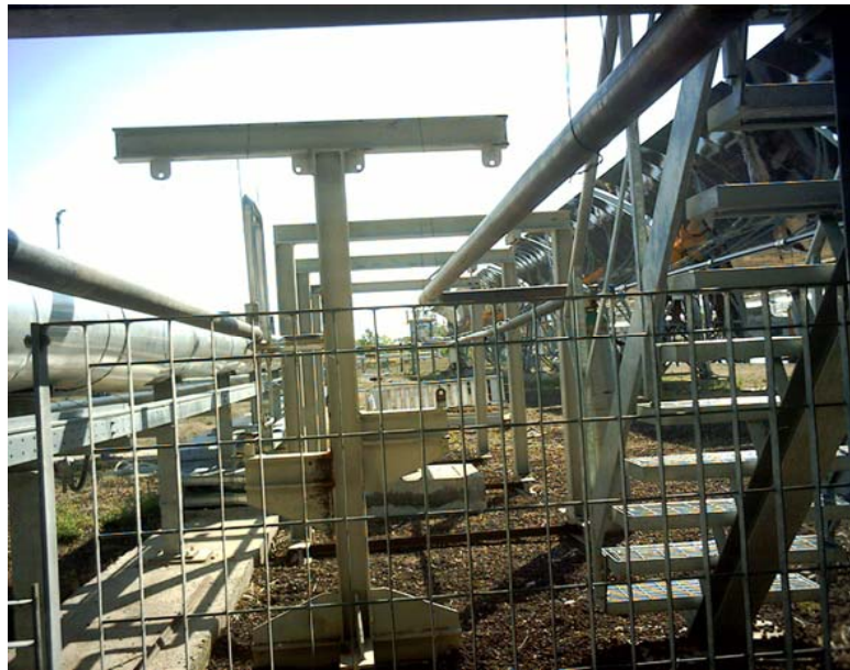
Piping without insulation
