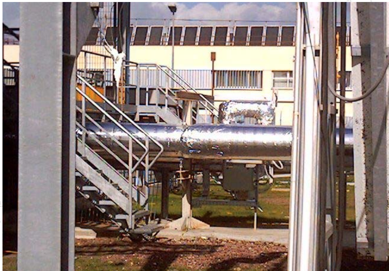
Piping with complete insulation
