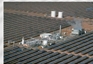
Parabolic Trough Rankine Cycle Power Plant
