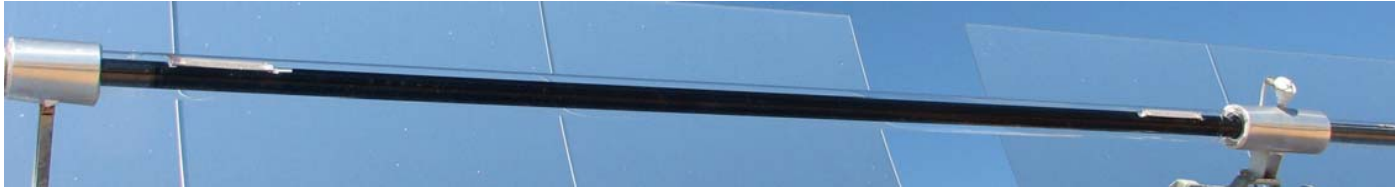
Visible Image of Receiver – Not Tracking
