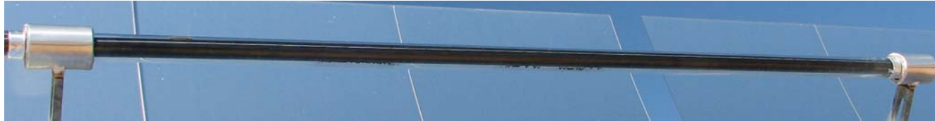
Visible Image of Receiver – Not Tracking
