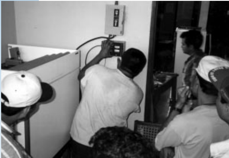
Figure 4.3. A photovoltaic technician's course completes the final installation checklist prior to commissioning a photovoltaic powered refrigerator/freezer at Clinica in the community of Mulukuku, Nicaragua.
