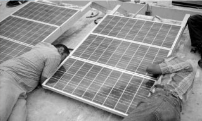
Figure 5.3. Technicians install photovoltaic panels on the roof of Clinica El Molino, near Trujillo, Peru.
