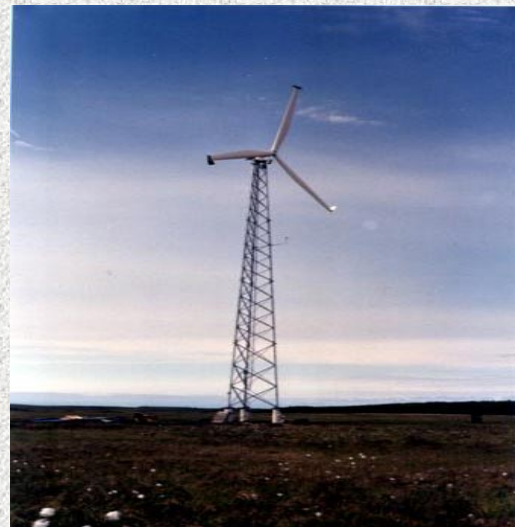
Atlantic Orient Corporation 50-kW wind turbine provides power to the Alaska Kotzebue Project.
