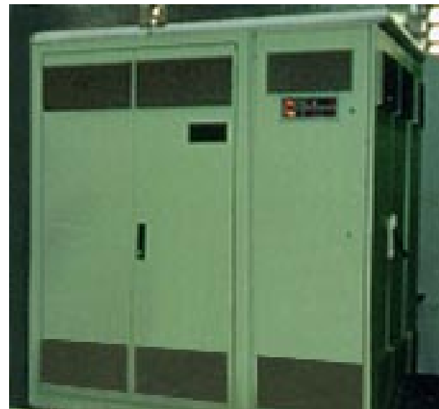
Prototype 25 kW SOFC in operation at the National Fuel Cell Research Center at Irvine, California. ETS is a founding member.
