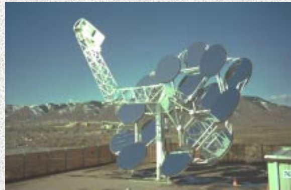
SAIC's 2 nd Generation 25-kW Hybrid Dish/Stirling System at Golden, Colorado
