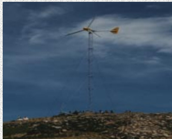
Wind water pumping station installed in Llasaraya, La Paz
