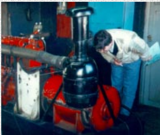
An isolated diesel plant in Tres Lagos, where a wind-diesel retrofit is under development
