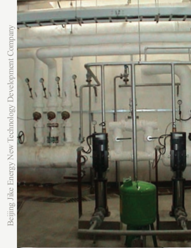
An interior look at the system that services 501 units in the Beijing Concordia International Apartment Building.
