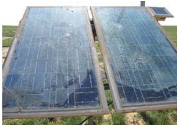
Badly damaged PV panels.
