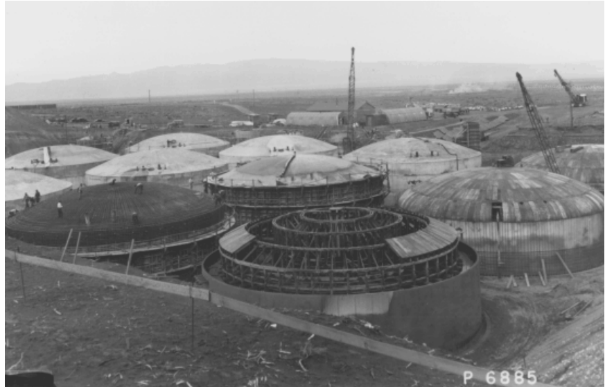
Hanford Single Shell Tank Farm Under Construction Circa 1944 (Source: DOE Integrated Management Plan for the Hanford TWRS, January 1999)
