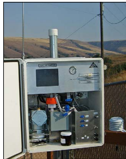
Air Monitoring Station
