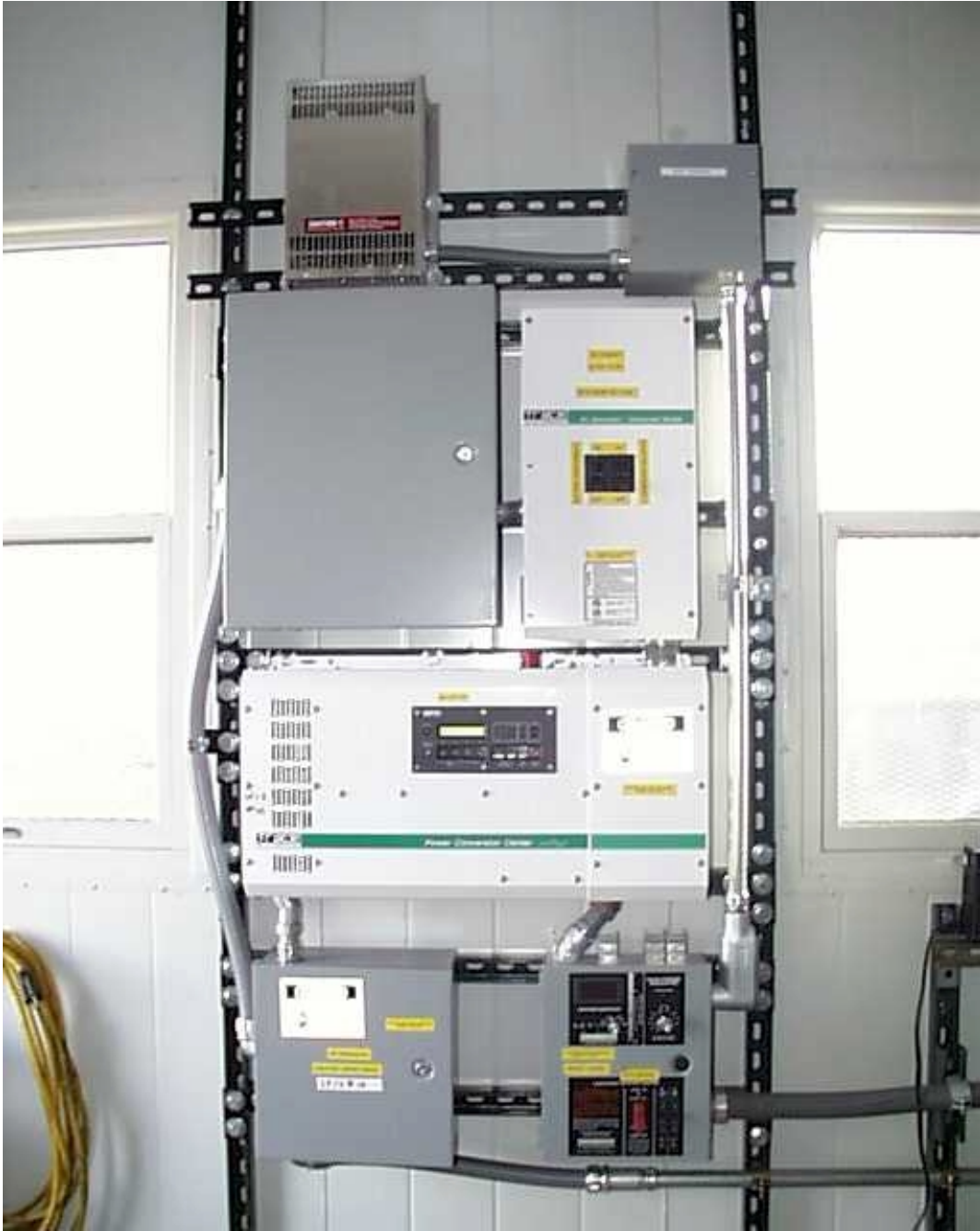
Figure 4. Photograph of Site 1.3 Electrical Installation
