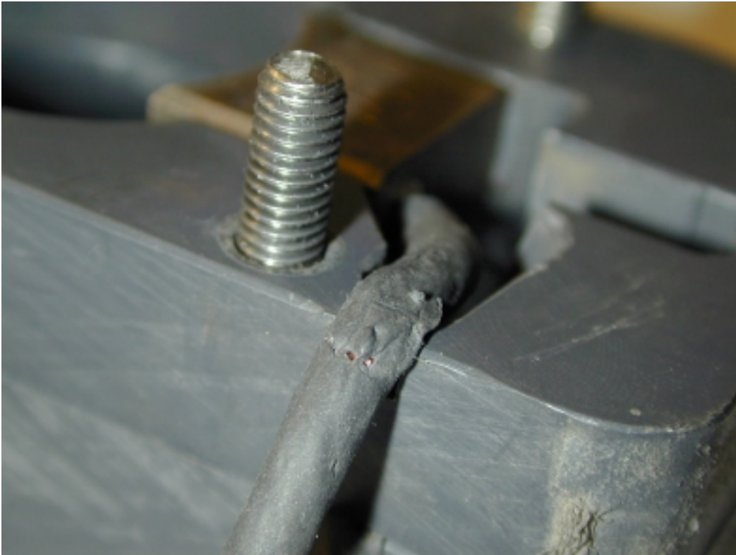
Figure 8: Damaged insulation on one of the wires coming out of the slip ring assembly.
