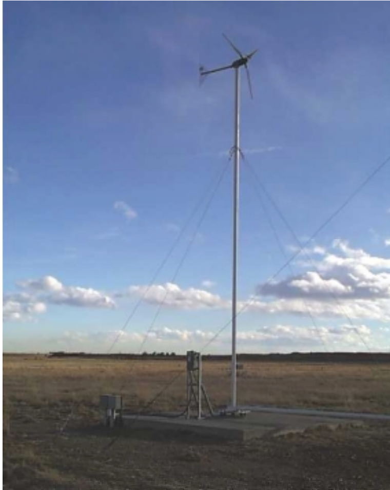
Figure 1. Overall Configuration of the Test Turbine, the Whisper H40
