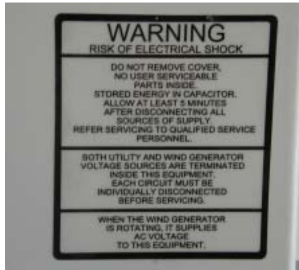
Figure 10: Warning sticker on the inverter.
