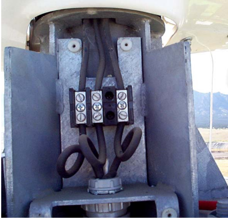
Figure 7. The up tower terminal strip.
