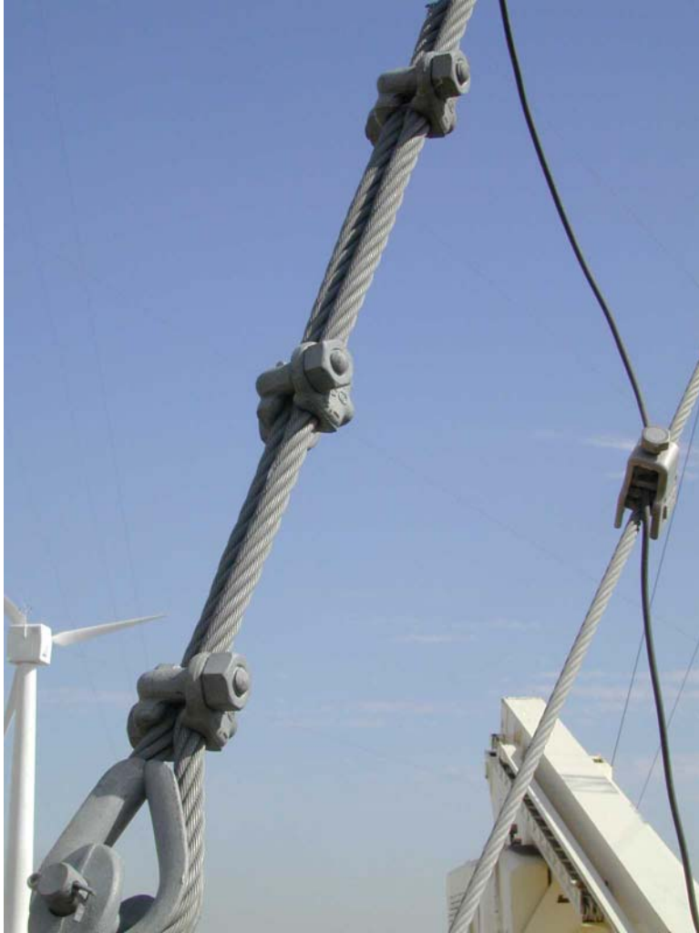
Figure 2. The wire clamps on the top west guy wire.
