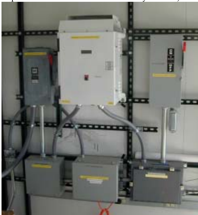
Figure 1. Overview of the turbine system inside the data shed. The Gridtek 10 inverter is in the center with disconnect switches to the turbine and the grid on either side. The boxes on the bottom are for NREL instrumentation.
