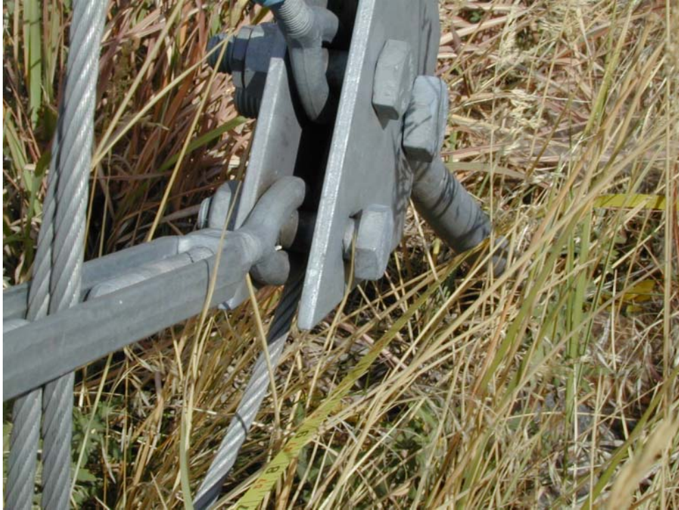
Figure 5. Equalizer plate on north guy anchor. Note that the bolt of the bottom guy wire is not secured all the way.
