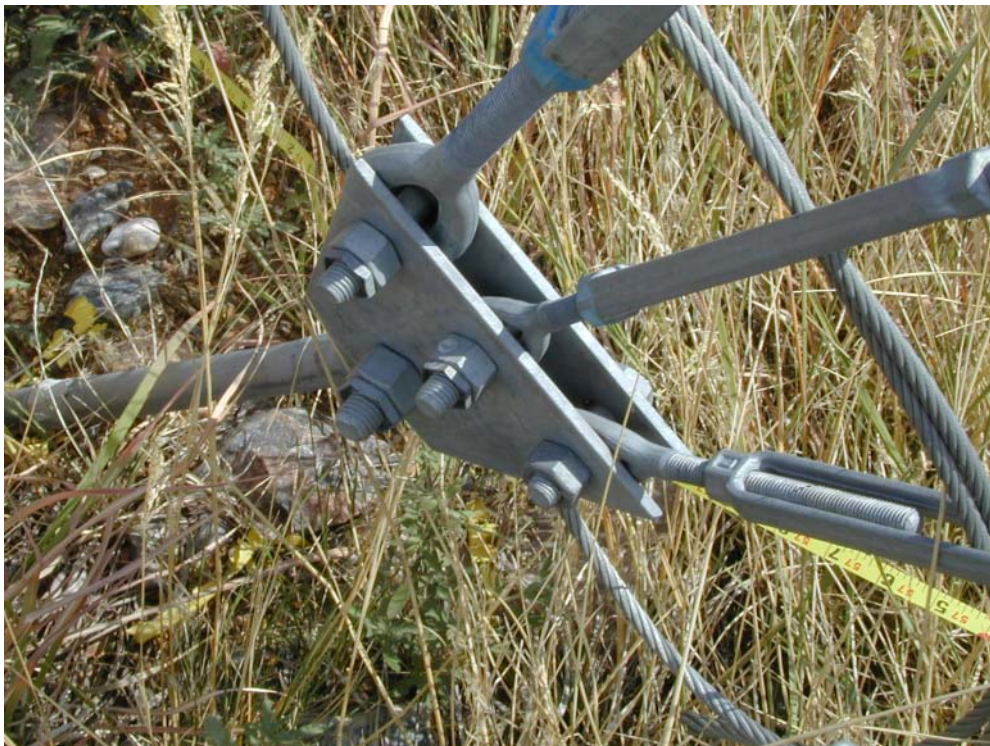
Figure 4. Close up of the equalizer plate on the north guy anchor. Note that the bottom guy wire does not have a lock nut.
