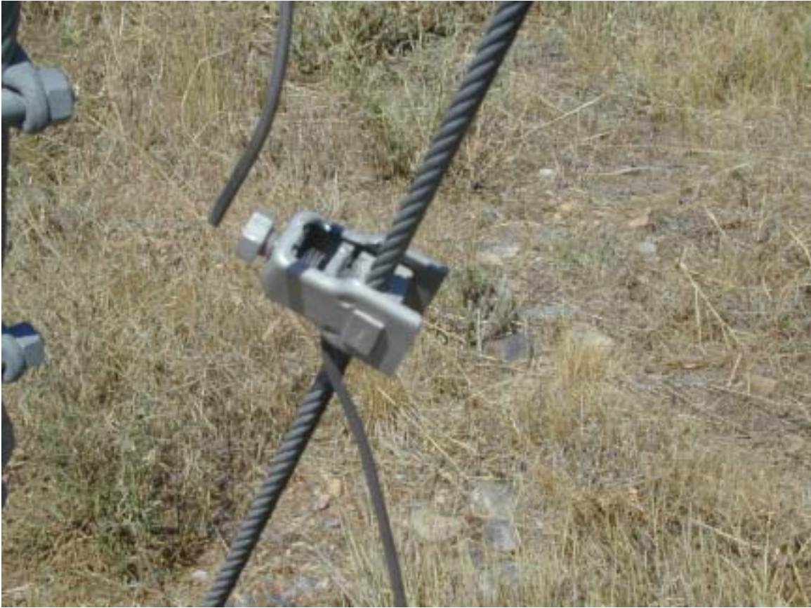
Figure 2. Broken ground wire at the top west guy wire.
