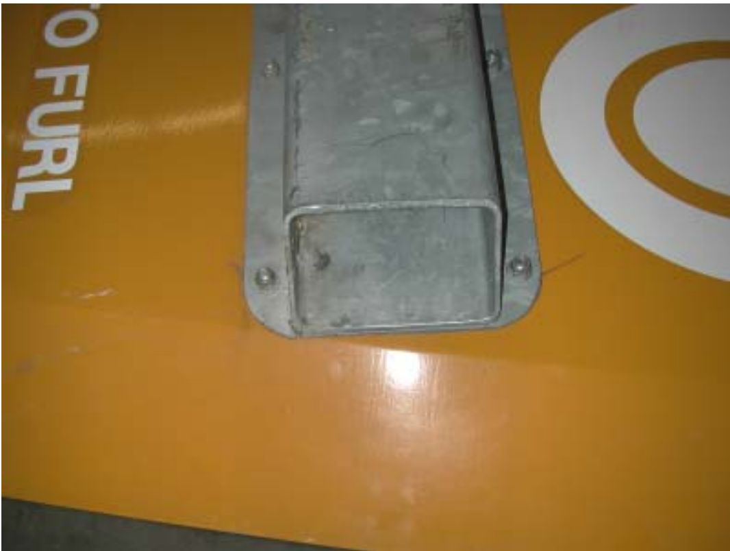
Figure D.7. Same cracks as in Figure 6, seen from other side.
