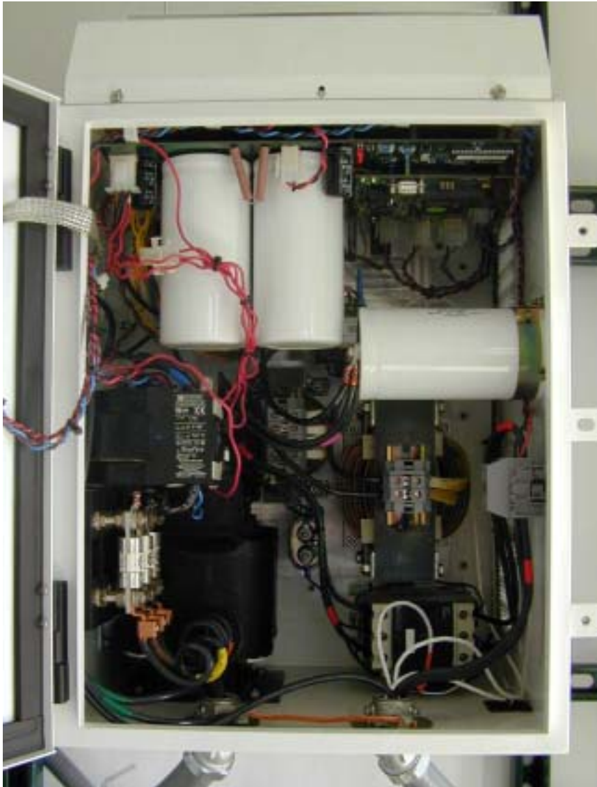
Figure 2. Overview of the inside of the inverter.
