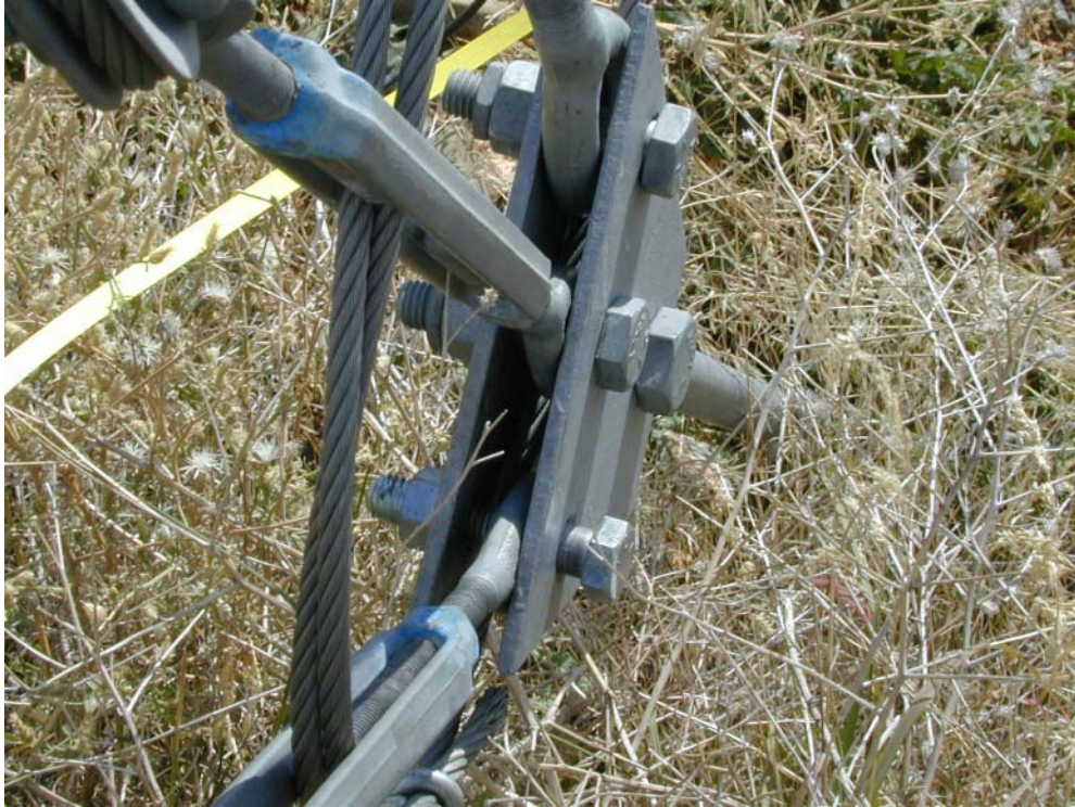
Figure 3. The southeast anchor point. Note that the bolt of the bottom guy wire does not have a lock nut on it and the nut is not tightened.
