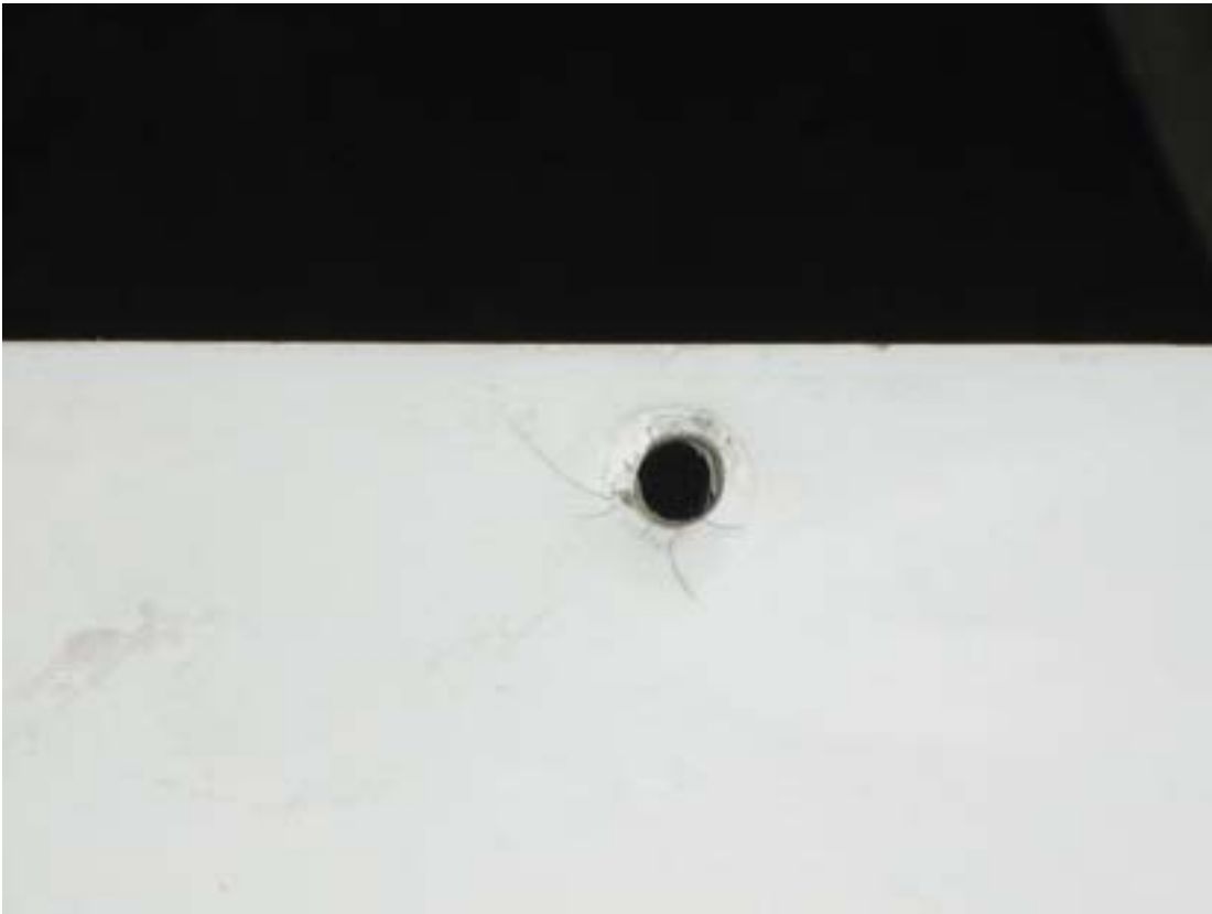
Figure D.5. Cracks near a bolt hole on the nacelle cover.
