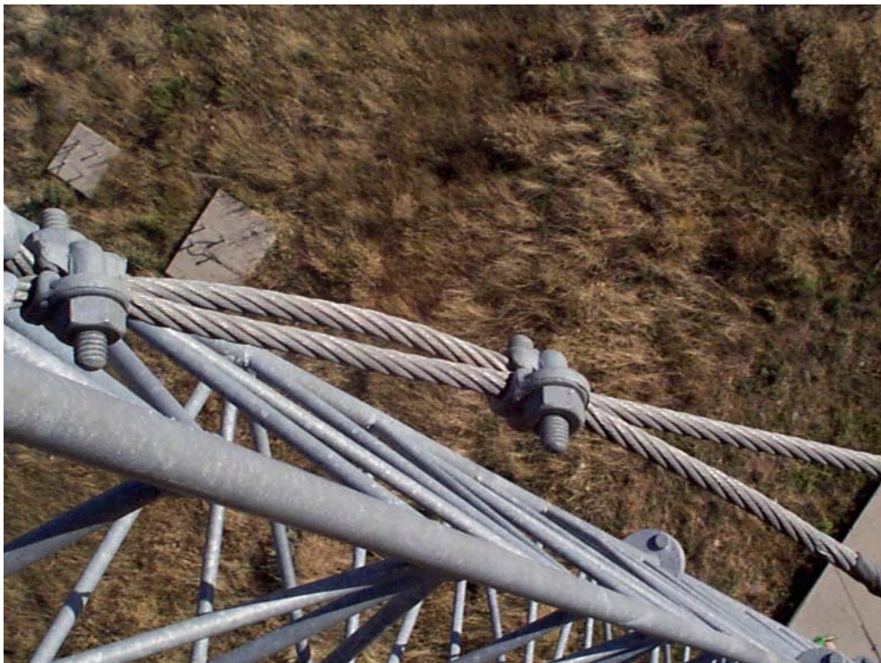
Figure 6. The western middle guy wire connection to the tower.
