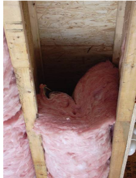
Figure 3.2.2 – Insulation settling away from sub-floor
