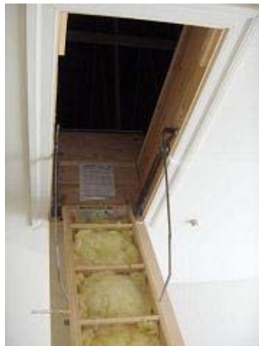
Figure 5.2.2 - Improperly installed insulation is compressed and impedes the use of the drop-down attic access stair.
