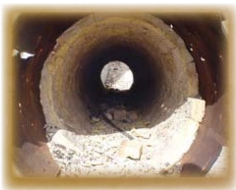
Eroded concrete water pipe
