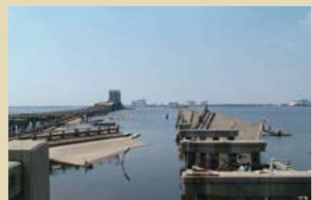
Hurricane Katrina damage to U.S. Highway Bridge.
