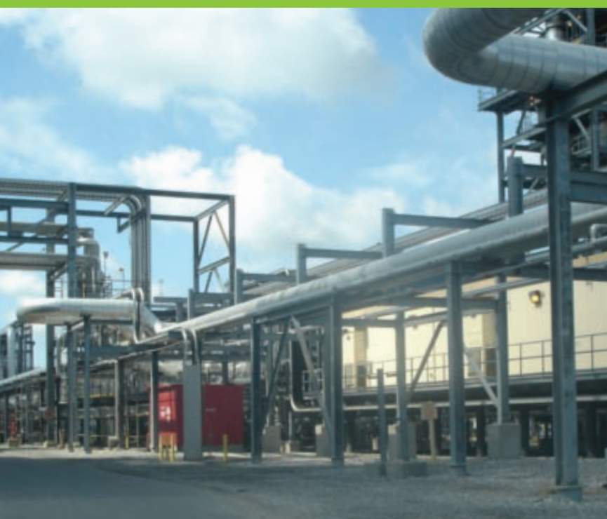
A utility pipe rack at Dow Chemical's St. Charles Operations in Hahnville, Louisiana.
