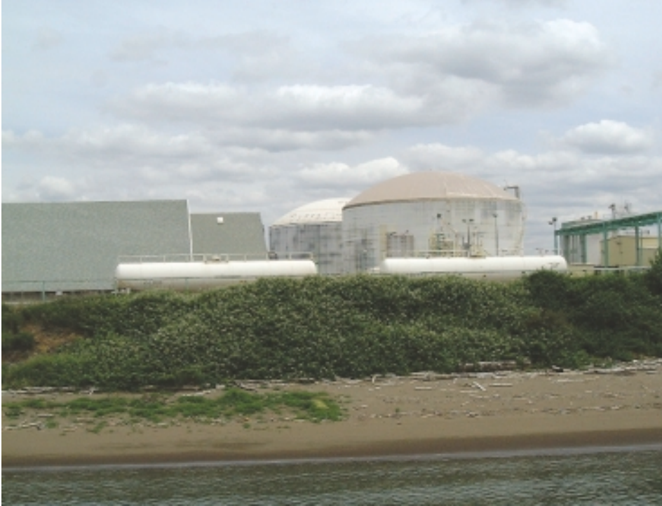
Ammonia Storage Tanks at the J.R. Simplot Rivergate Facility in Portland, Oregon
