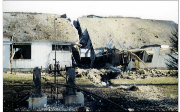
Damage caused by impact of large tank fragments
