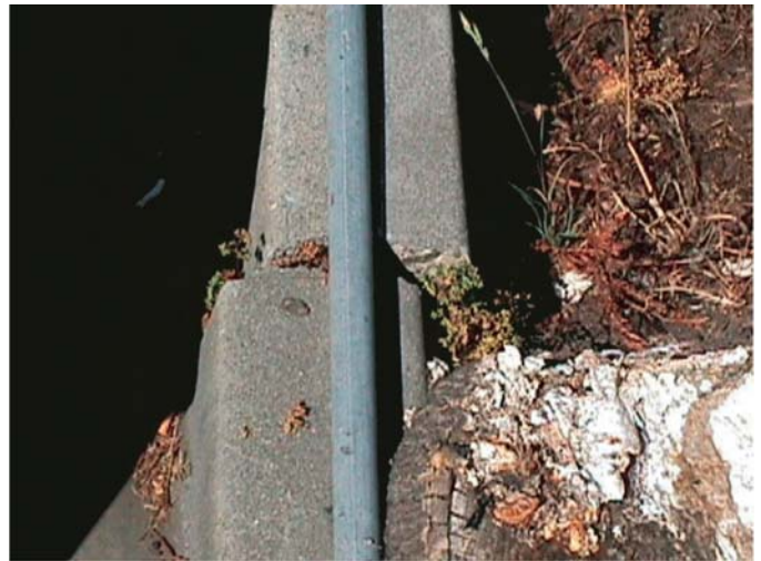
Figure 45. Photograph of evidence of right lateral creep on the mapped active strand of the Hayward fault. This offset curb is in the parking lot between A and B streets in downtown Hayward.
