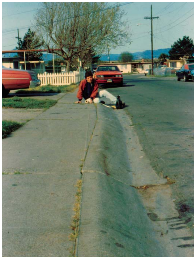
Figure 24. Right-lateral curb offset at 704 Phanor Drive due to aseismic slip in Parchester Village that was 150 mm (6 inches) by 21 March 1985. More precise techniques found 214 mm of offset in a wider span of the northwestern curb on Banks Drive in 1988 (Lienkaemper et al., 1991). By now, the offset should be about twice as much as shown here. Gene Kelley, Colorado State University, for scale.
