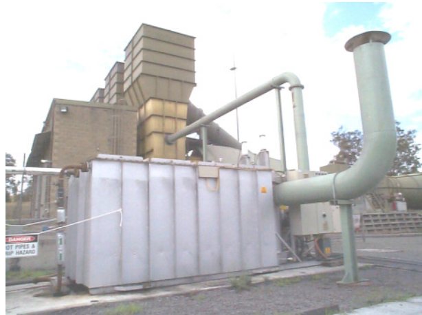
Ventilation air methane equipment (Megtec Vocsidizer) in Australia. (Courtesy of BHP Billiton Ltd.)
