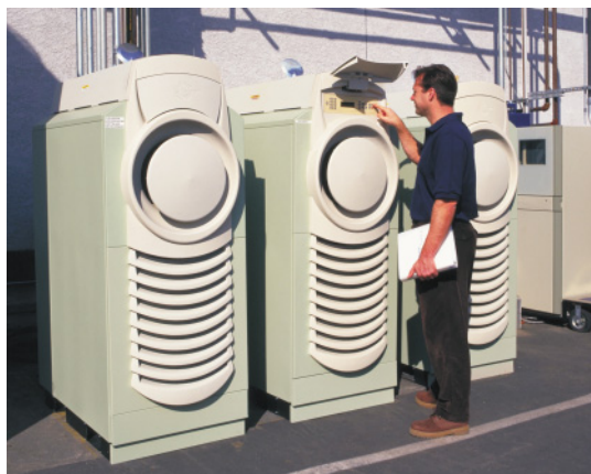
Three 30-kW microturbines are in use at a landfill in Burbank, California, to generate electricity.
