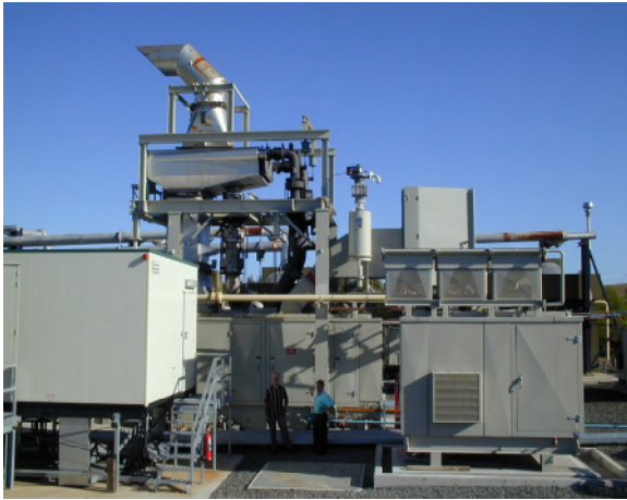
Lean fuel turbine running off of ventilation air methane and drained gas. (Courtesy of Energy Developments Ltd.)
