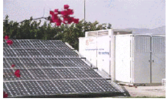
Hydrogen production by photovoltaic hydrolysis.
