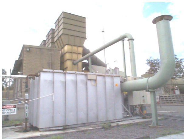
Ventilation air methane equipment (Megtec Vocsidizer) in Australia. (Courtesy of BHP Billiton Ltd.)
