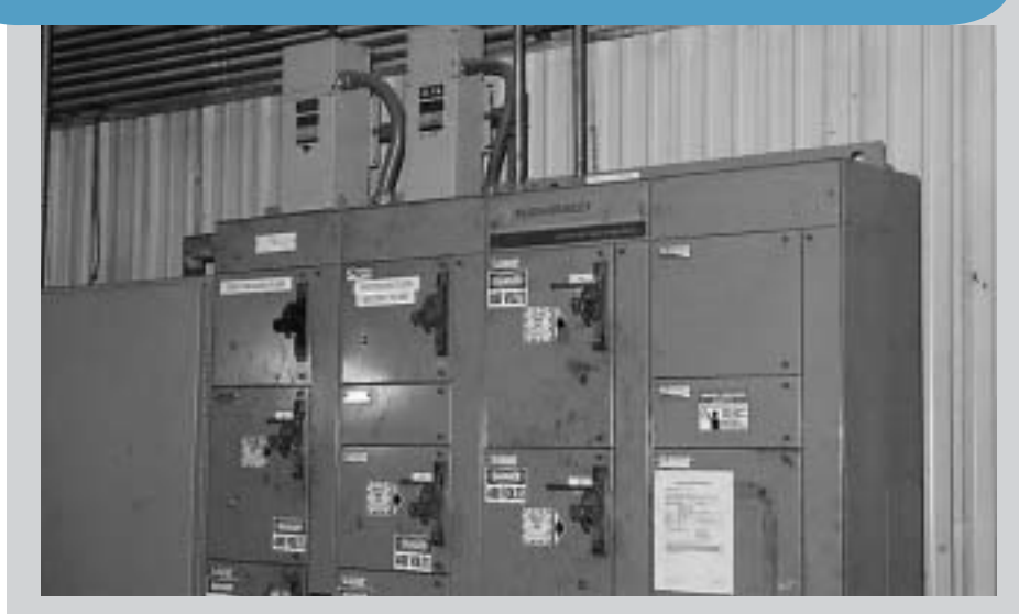
CAPACITORS INSTALLED AT LOMA SAW MOTOR CONTROL CENTER
