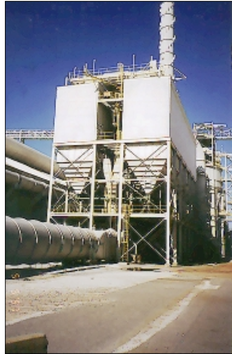
Pot Line Dust Collector
